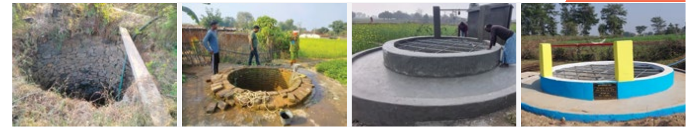
(Left to right) Wells before and after intervention in Khaira block - Jamui, Bihar
