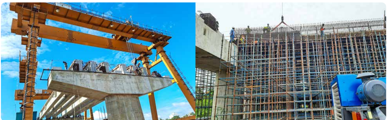
▶ Project Management Consultancy for the Ashuganj Akhaura Land Port Road as a four-lane National Highway Project in Bangladesh
