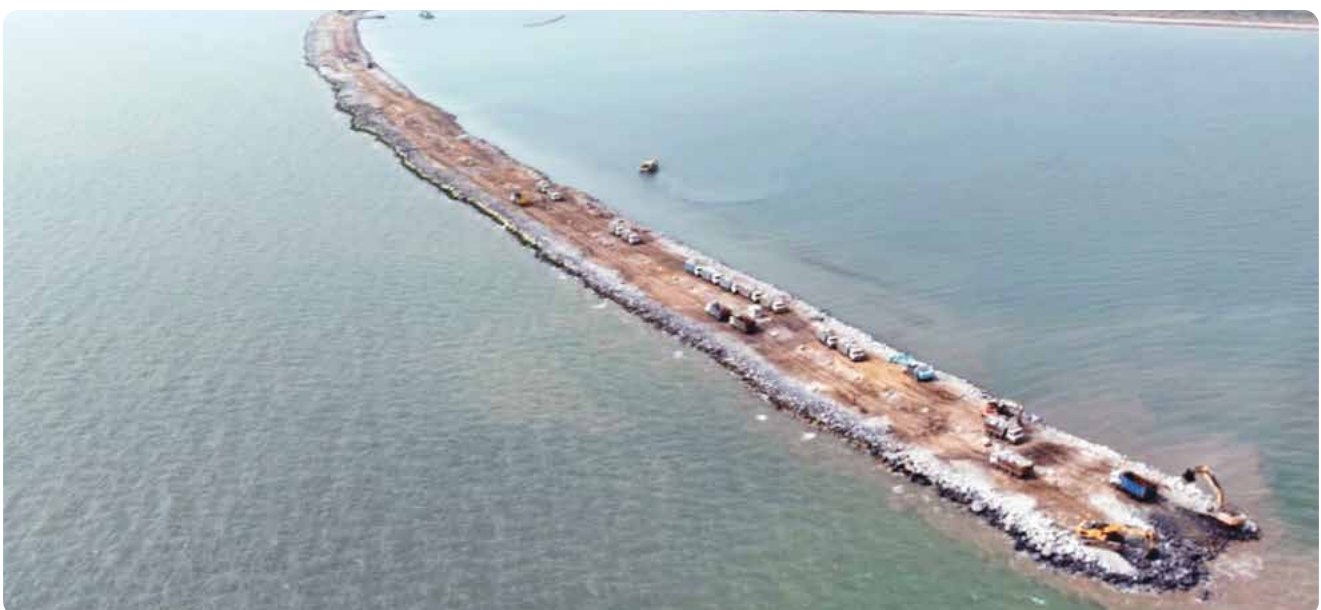
▶ Project Management Consultancy for the development of a greenfield port at Machilipatnam
