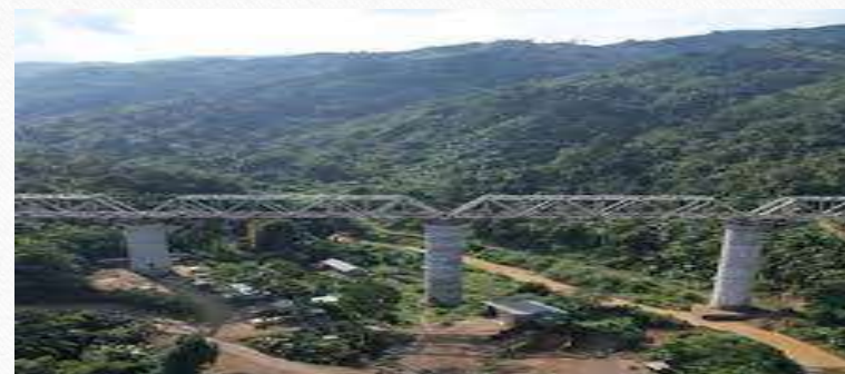
Construction of foundation and sub structure over pile foundation for Tall Bridge of new BG Railway line from Bairabi to Sairang (Mizoram).
