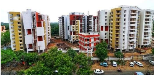
Construction of 222 Flats at Keelandev Tower, Bhopal for MP Housing & Infrastructure Development Board
