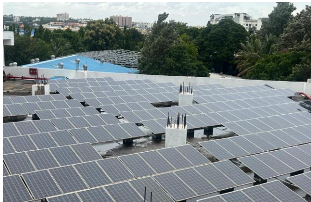
Solar Panel Projects continue with three more plants going live in FY24
