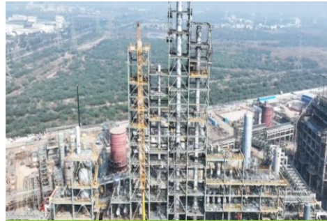
MIBK & MIBC plant
