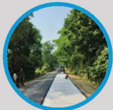
Laying of Paving fabric and Providing BC / PQC over the stabilized Layer
