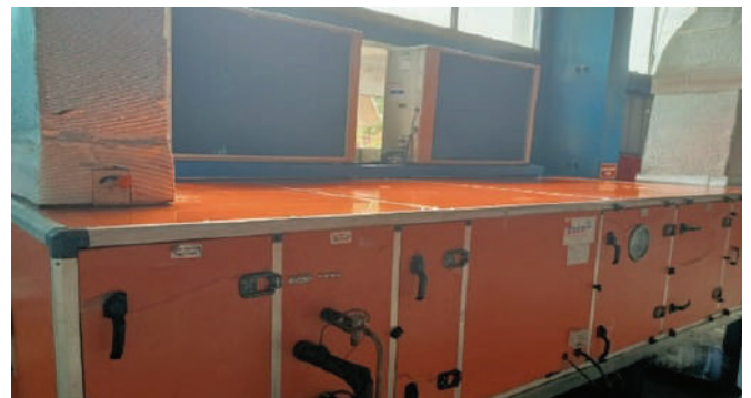
Efficient HVAC system - AHU systems
