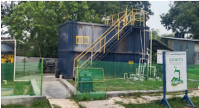
Wastewater Treatment plant
