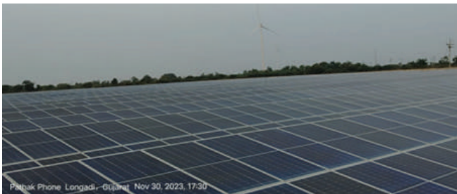
10 MW Wind Solar Hybrid plant
