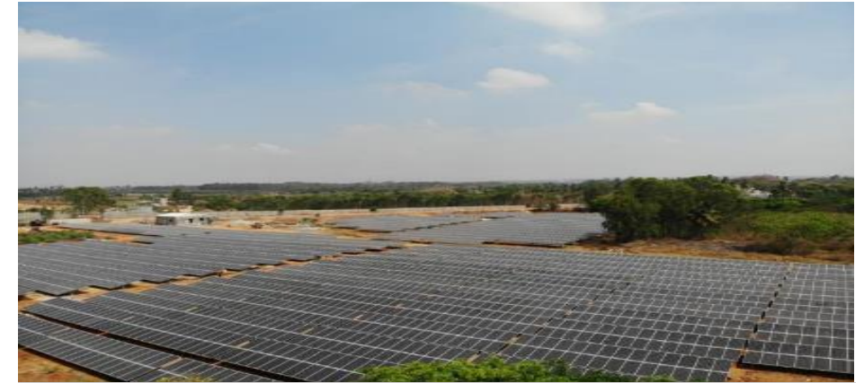
Solar Panels at HRGRDC, Bengaluru
