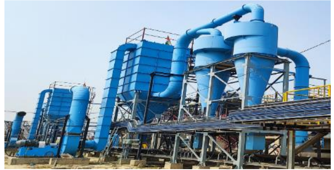
CBG Plant at Budaun- Milling Section
