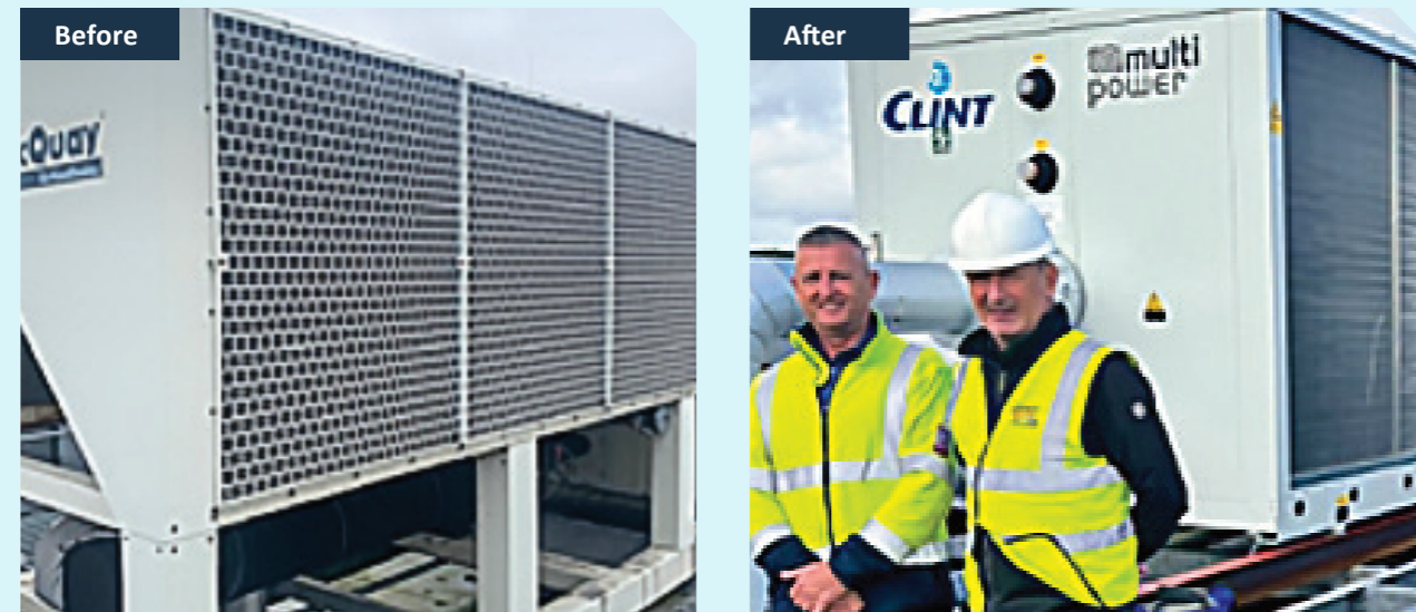
Upgraded High Efficiency Chiller, Morpeth, UK
