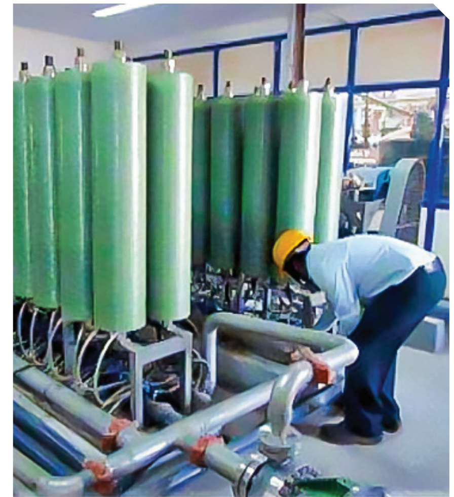
➤ Reverse Osmosis (RO) plant, Digwal, India
