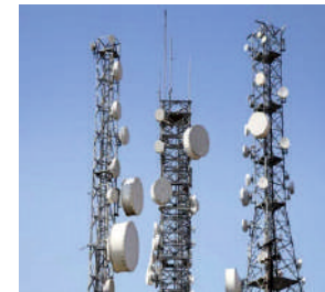
5G Telecom Towers
