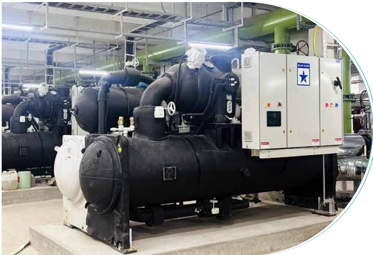
MEP works done by Blue Star at Tata Electronics, Hosur, Tamil Nadu
