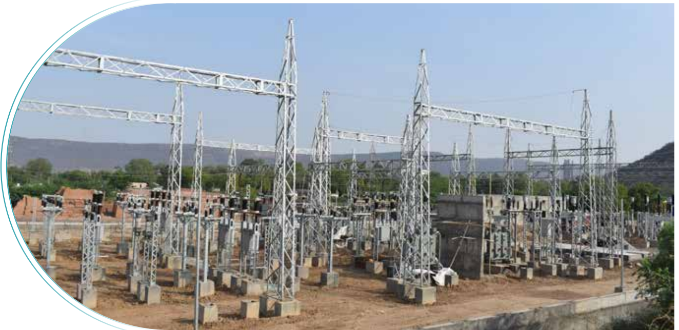
Railway Electrification - Traction Sub Station at Lakheri, Rajasthan
