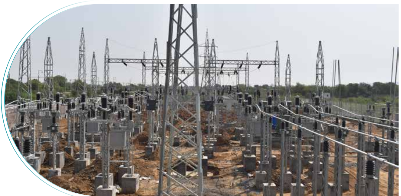
Railway Electrification - Traction Sub Station at Sawai Madhopur, Rajasthan
