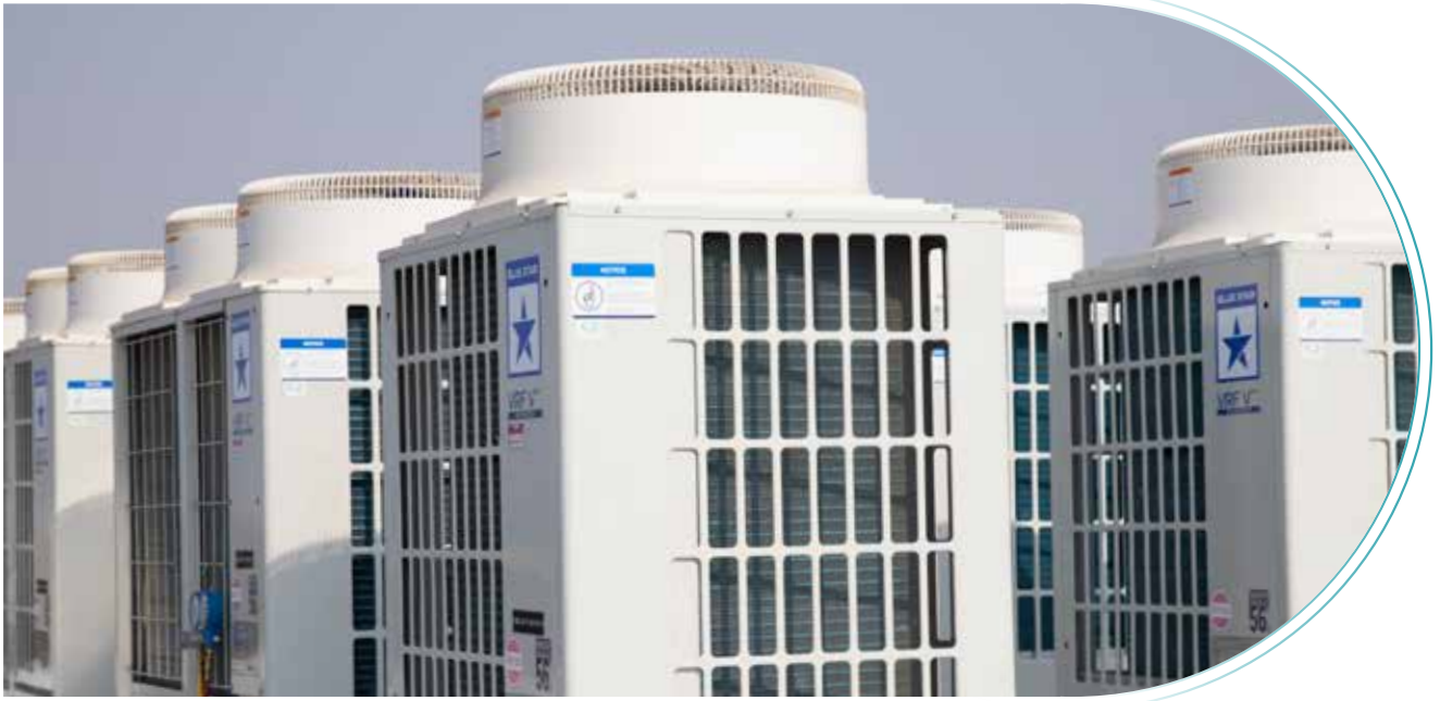
VRF system installed at STT, Pune
