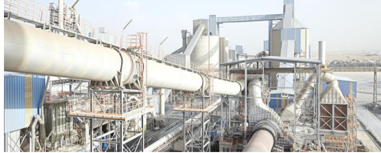
Electricals control and implementation package for a cement clinker and waste heat recovery system
