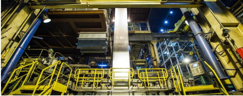
Motors and drives package for a hot strip mill with continuous galvanizing line of a major global steel manufacturer
