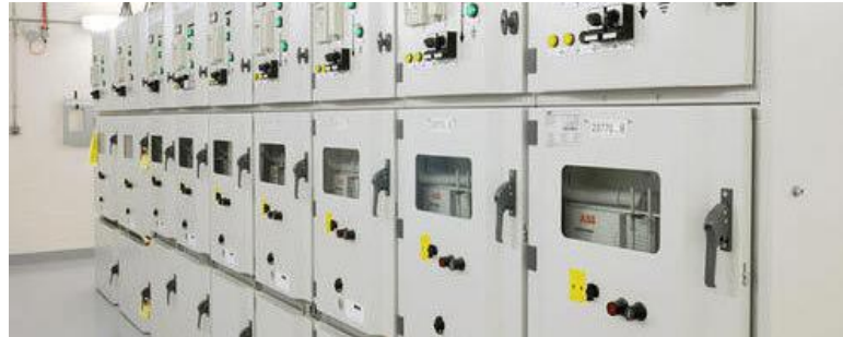
Power distribution equipment like switchgears for a leading metals major
