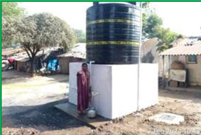
Providing Borewell with Submersible motor and PVC tank with platform at Village Shah (Navapara), Taluka Mangrol, District Surat
