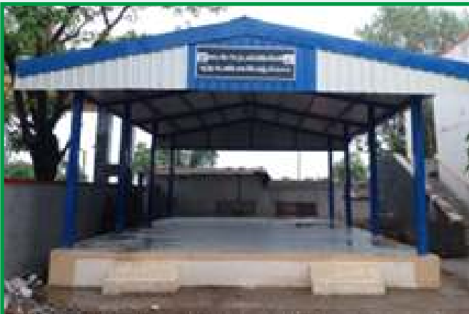
Construction of Multi-Purpose Shed for Primary School at Village Ushker, Taluka Mandvi, District Surat
