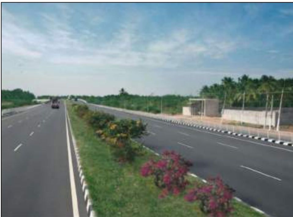
Figure 8-2 : General Condition of project road.
