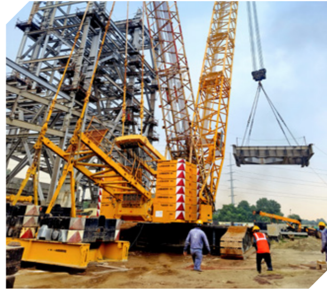
▶ Liebherr LR 1400-2 400 MT Crawler crane doing structure module frame erection at Baruni, Bihar - one of our EPC projects
