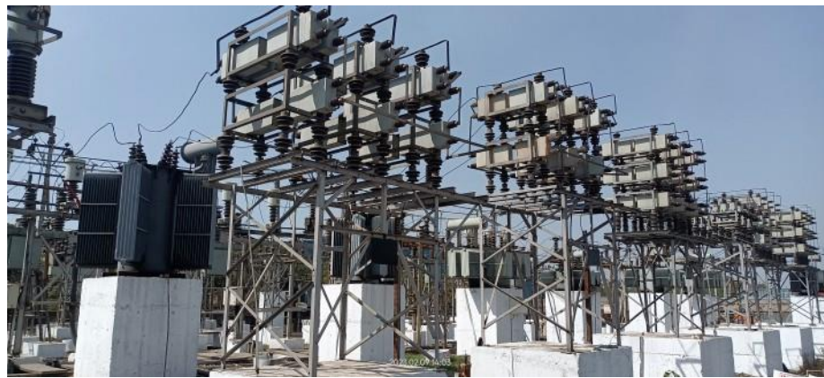
CosPower's Capacitor Banks Installed and in Service in a Steel Plant
