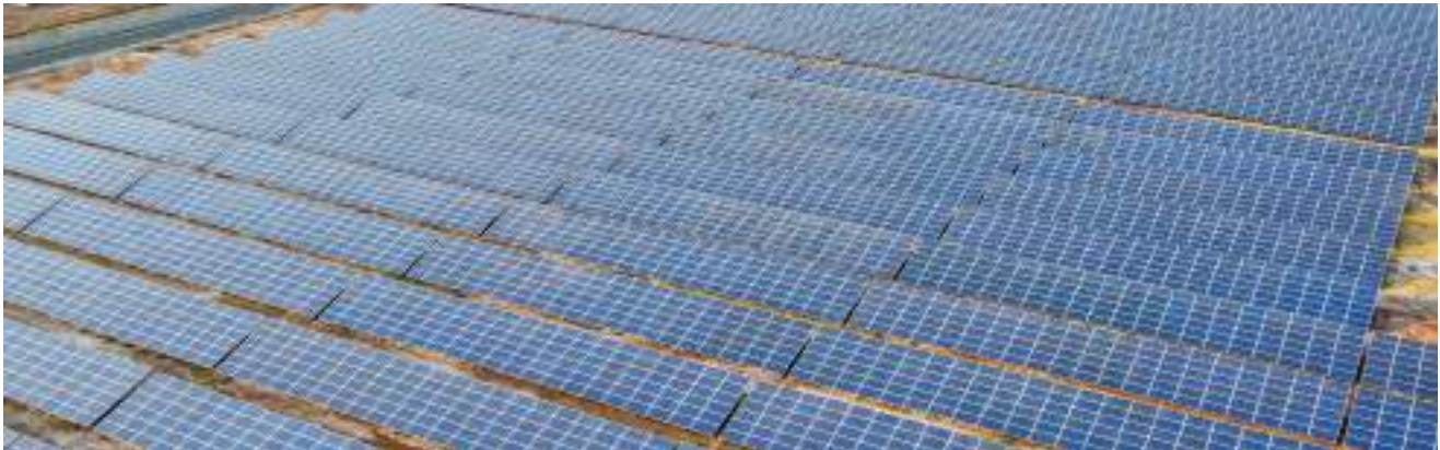
51 MW Solar Power Plant, Patan
