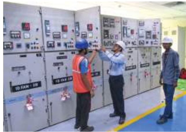
Control room at our Coal-based Plant
