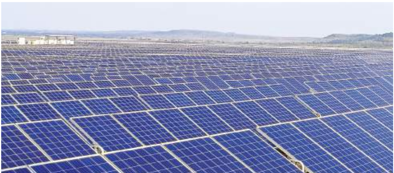
50MW Solar Power Plant at Telangana
