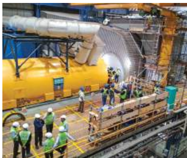
Turbine Floor at Gas-based Generation Plants, Surat
