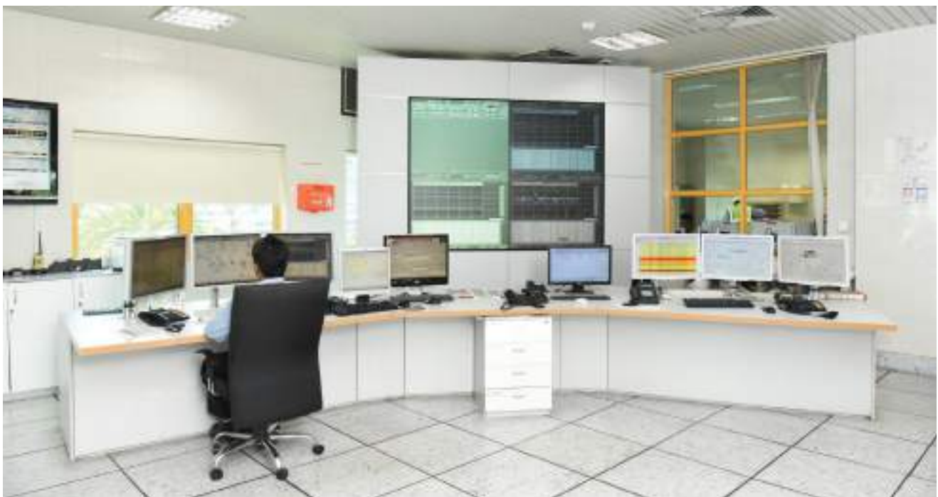
Monitoring Room at Gas-based Generation Units, Surat
