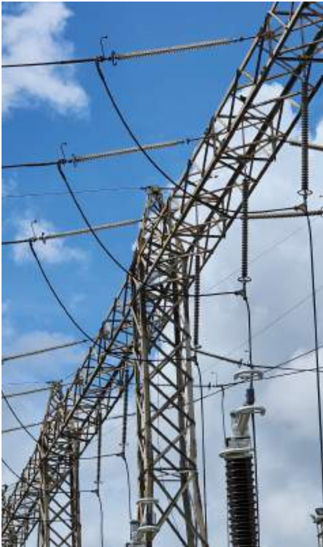
Polymer based insulation in Transmission Tower at Surat
