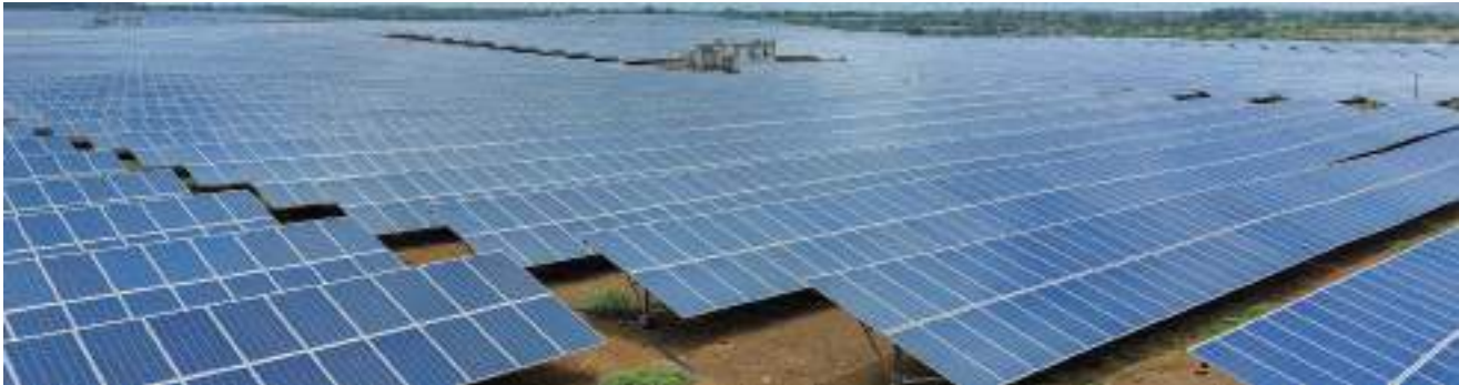
87 MW Solar Power Plant, Surat
