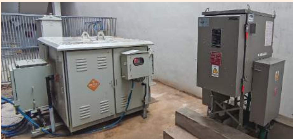
Distribution Transformer at Agra
