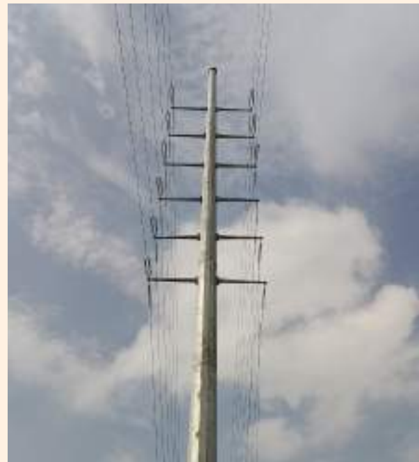
Monopole Tower at Ahmedabad
