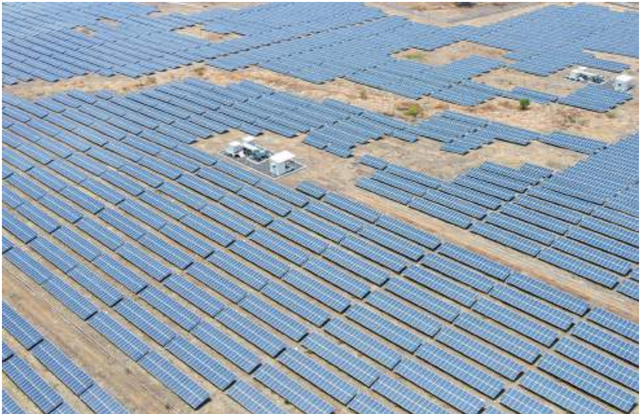
50 MW Solar Power Plant, Solapur
