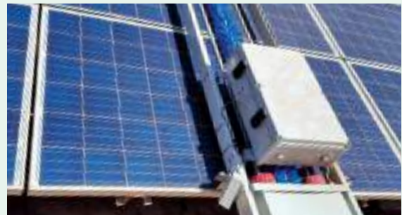
Cleaning of Solar Panels using Robots at Charanka Solar Plant
