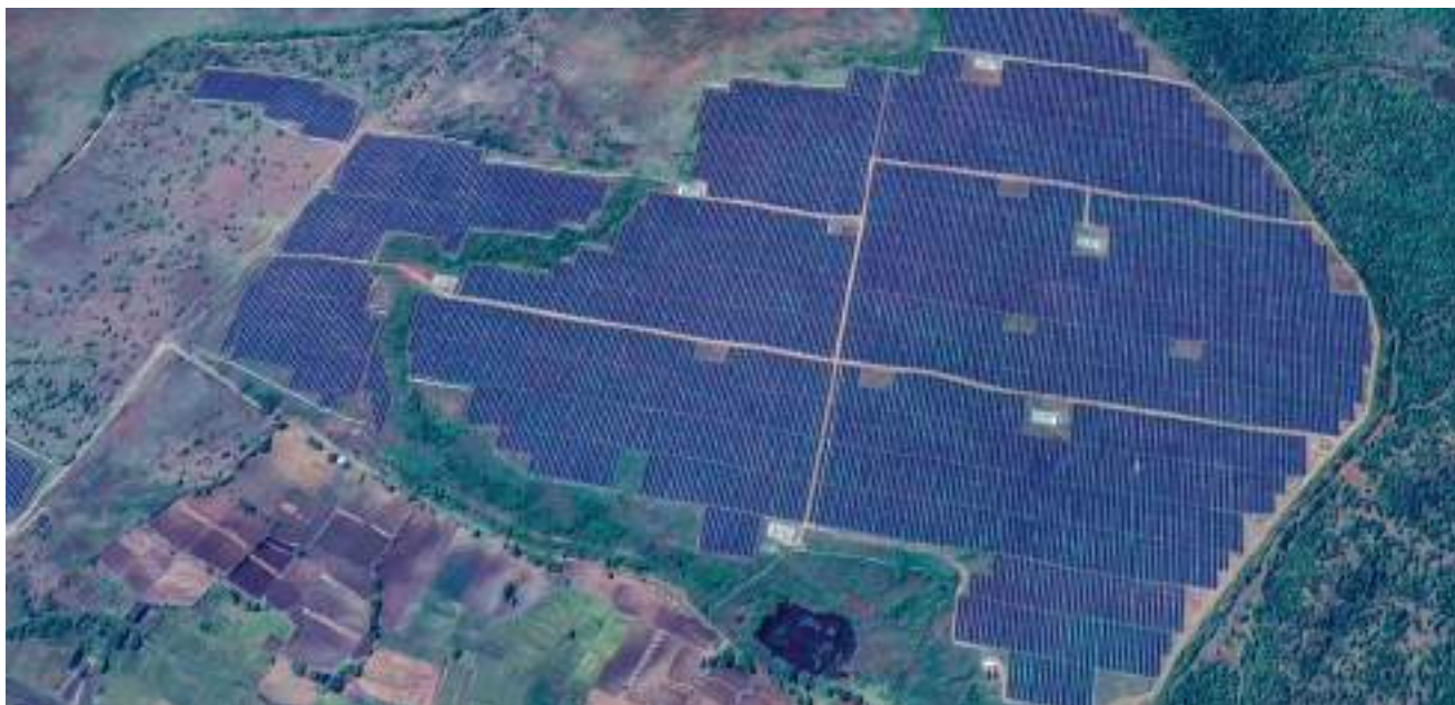
Aerial View of our 50MW Solar Power Plant at Telangana
