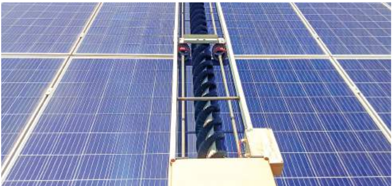
Cleaning of Solar Panels using Robots at Visual Solar Plant
