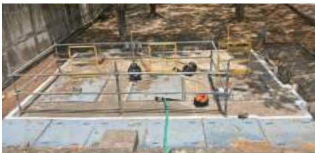
Rain Water Harvesting at SUGEN
