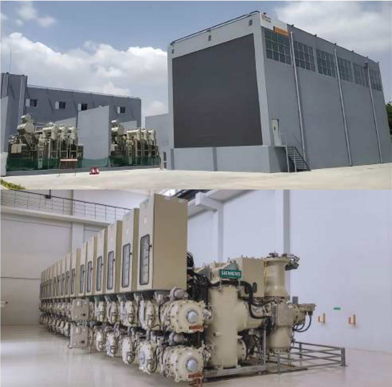
132 kV Gota Substation at Ahmedabad
