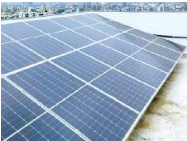
Solar Rooftop at Ahmedabad Distribution Unit
