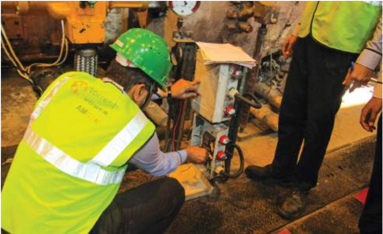
Maintenance activity at AMGEN Plant, Ahmedabad
