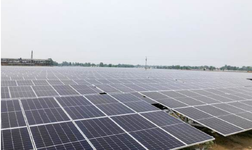
Offsite solar plant for Phoenix Palassio, Lucknow
