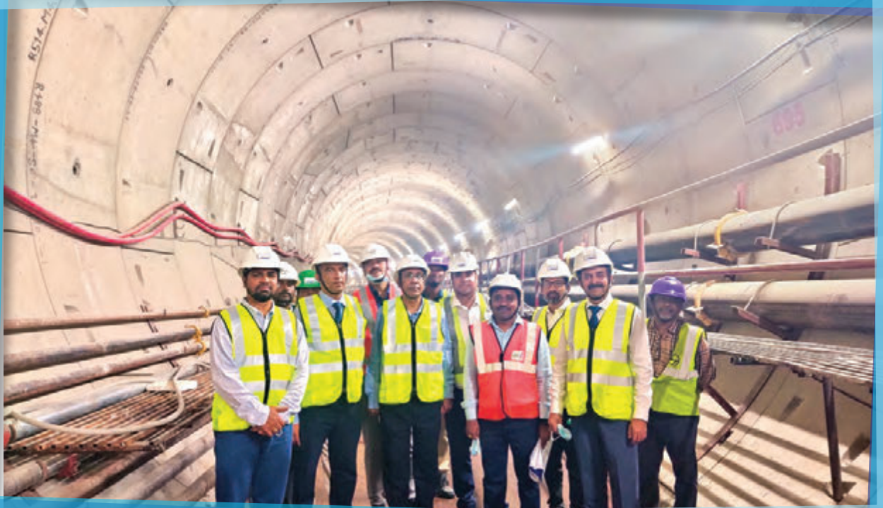
Tunnel Ventilation System (TVS) and Environmental Control System (ECS) works being executed by Blue Star for Bangalore Metro Rail Corporation
