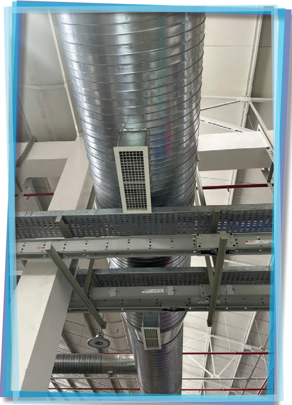
MEP works including HVAC works executed by Blue Star at the Freudenberg Plant, Morinda, Punjab
