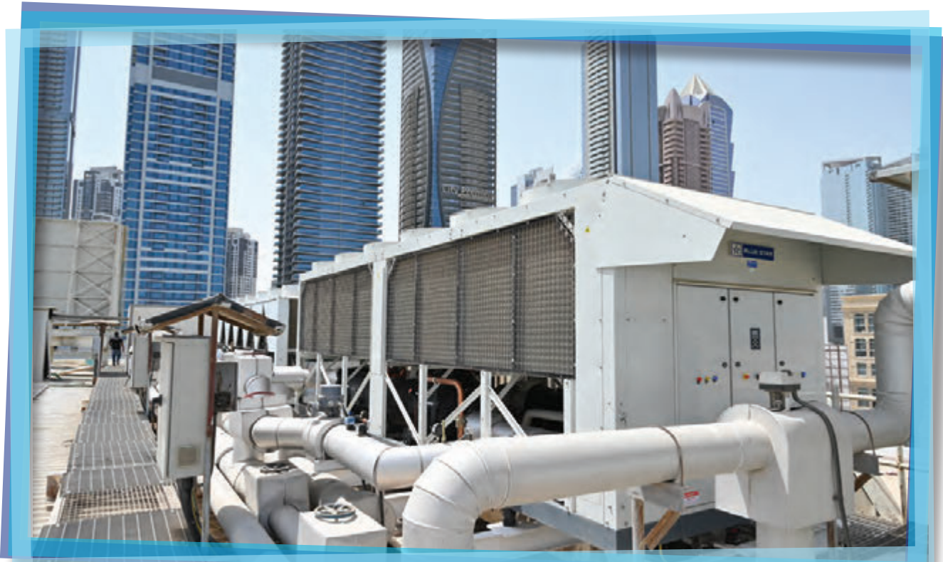
Revamp of Chillers executed for AL Rostmani Group - AL Wasl Shopping Centre, in Dubai
