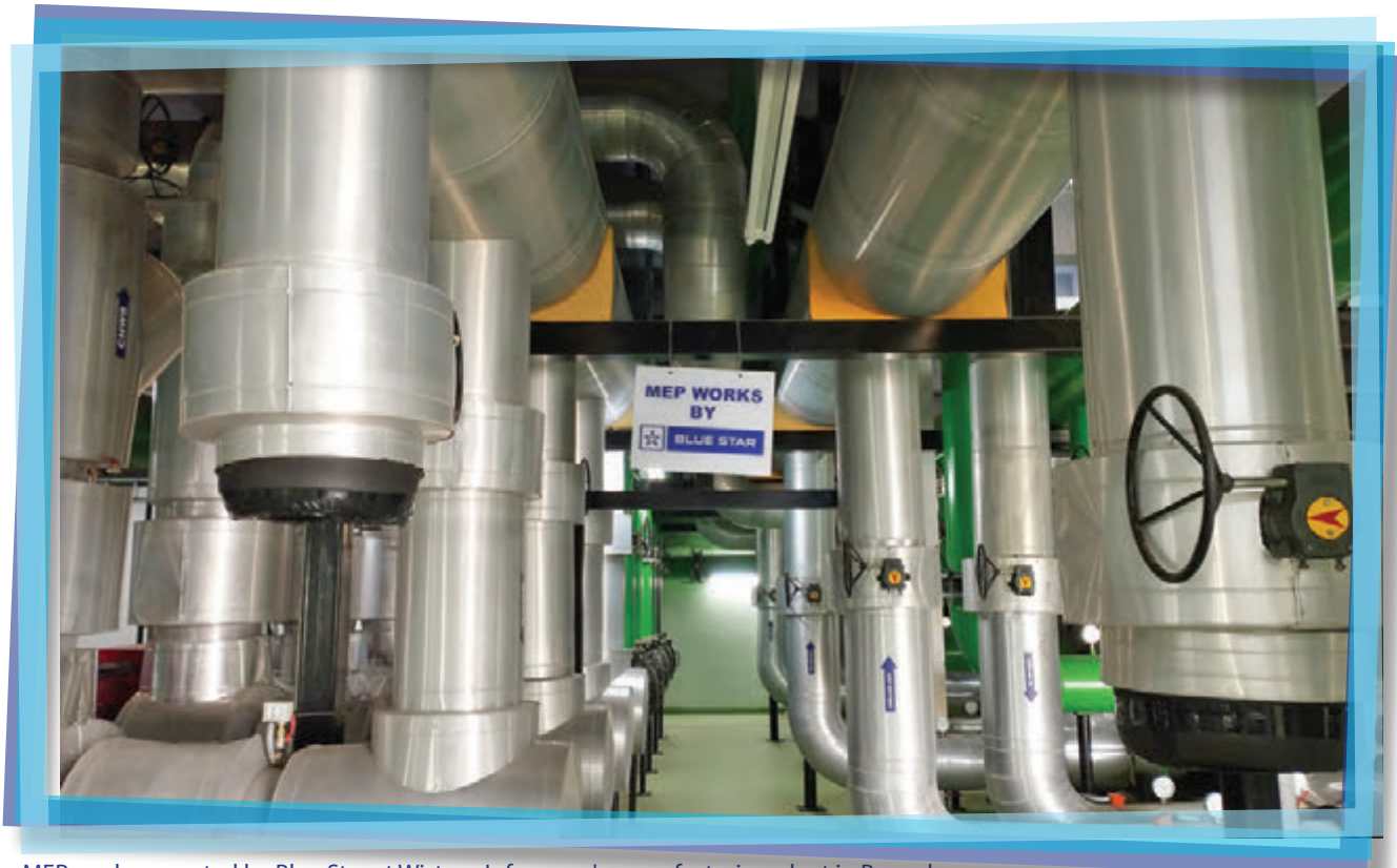
MEP works executed by Blue Star at Wistron Infocomm's manufacturing plant in Bengaluru
