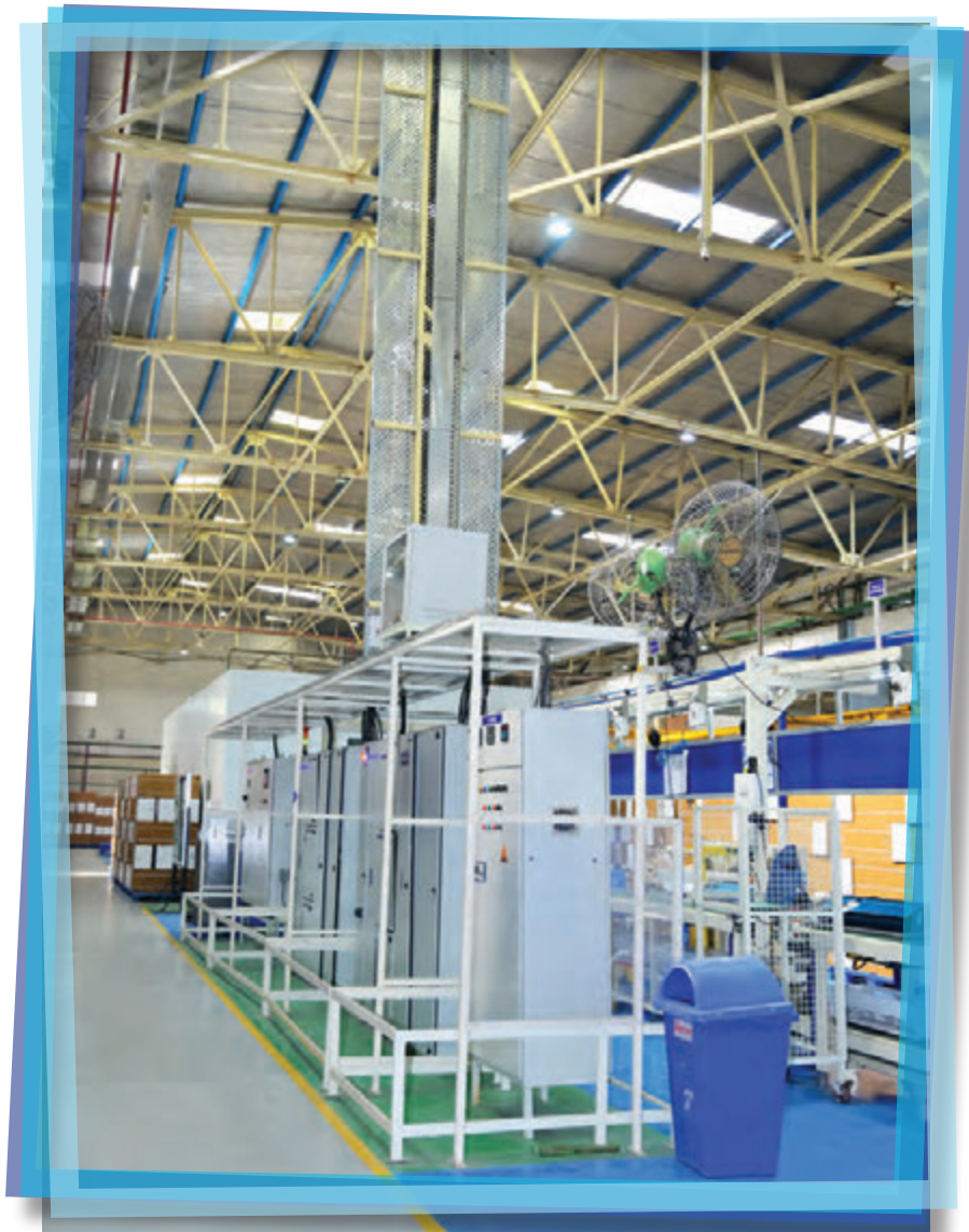
Centralised utility control panels of the indoor unit assembly line at Blue Star's Himachal Pradesh Plant
