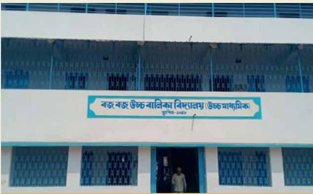
Restoration of School Building and facilities at Budge Budge Uchcha Balika Vidyalaya (H.S.) at Budge Budge
