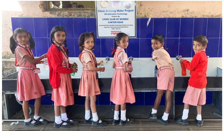
Clean drinking water project implemented by Anarde Foundation
