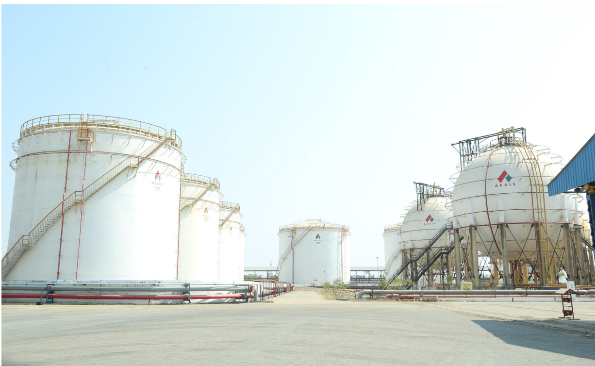
Liquid and LPG tanks at Pipavav terminal
