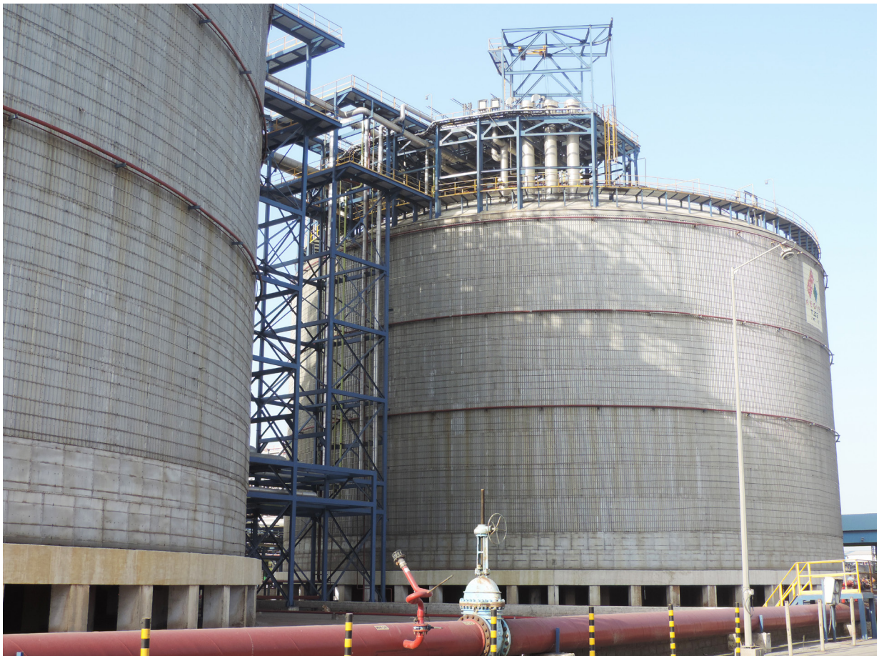
Close-up of LPG tanks at Kandla terminal
