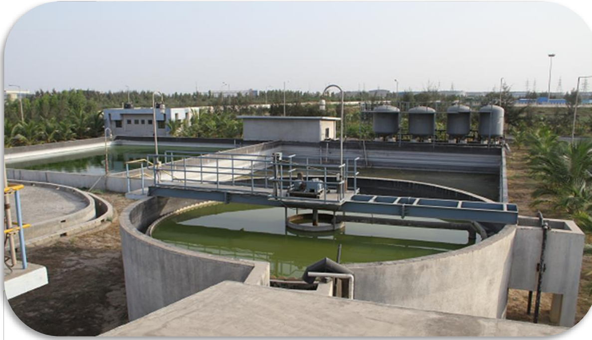
Water treatment plant at Mundra
