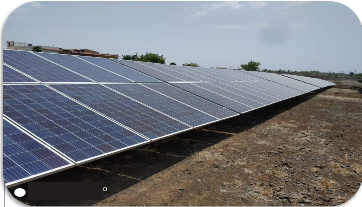
Solar Panel for Aux Power generation for Office use
