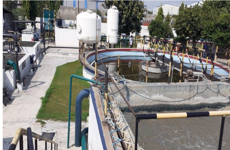
Greater Noida - Effluent Treatment Plant
