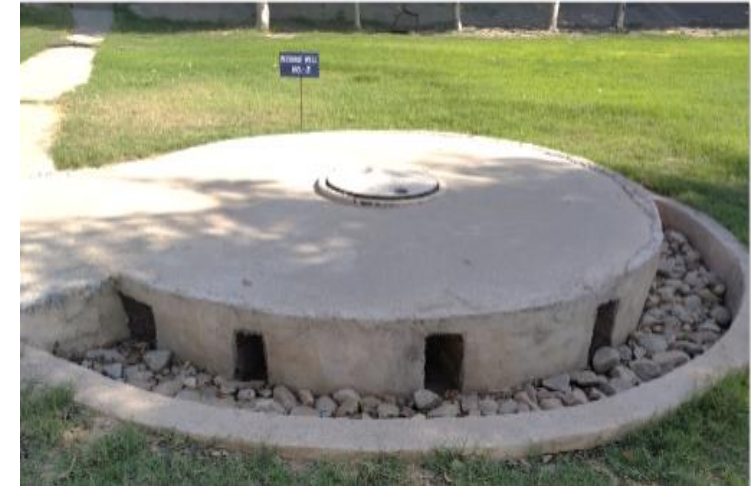
Bhiwadi - Rain water harvesting pit
