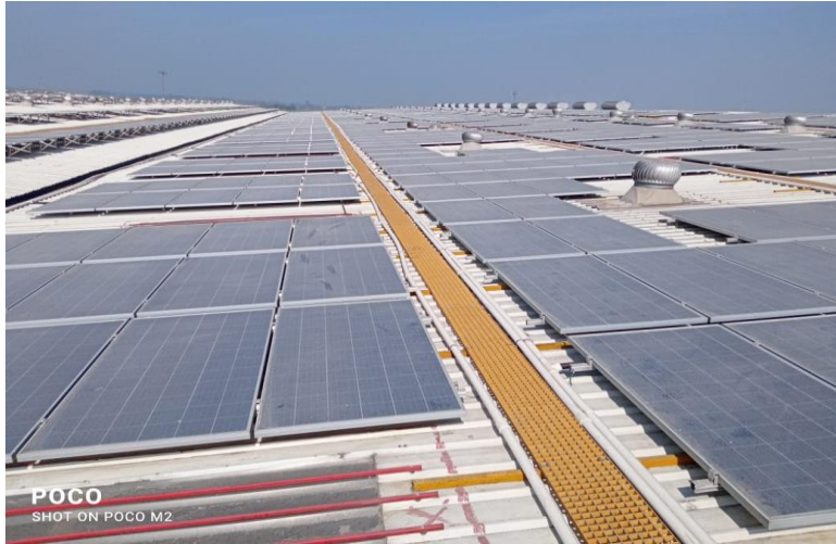
Sandila - Rooftop Solar Panels
