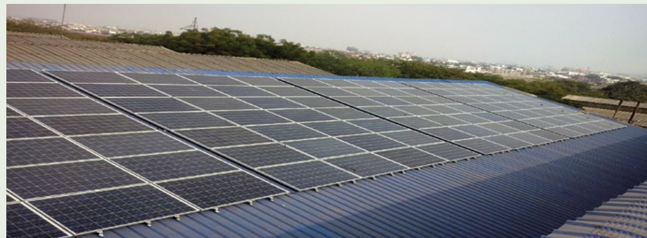
Solar rooftop power plant, Jaipur manufacturing unit
