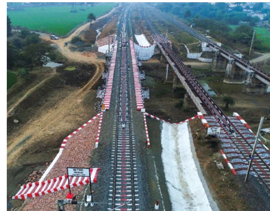
Bhopal-Itarsi Third Line project, Madhya Pradesh, comprising track laying, OHE, S&T works, bridges, stations and other railway infrastructure
