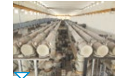
765/400 kV North Chennai Gas Insulated Substation, Tamil Nadu
