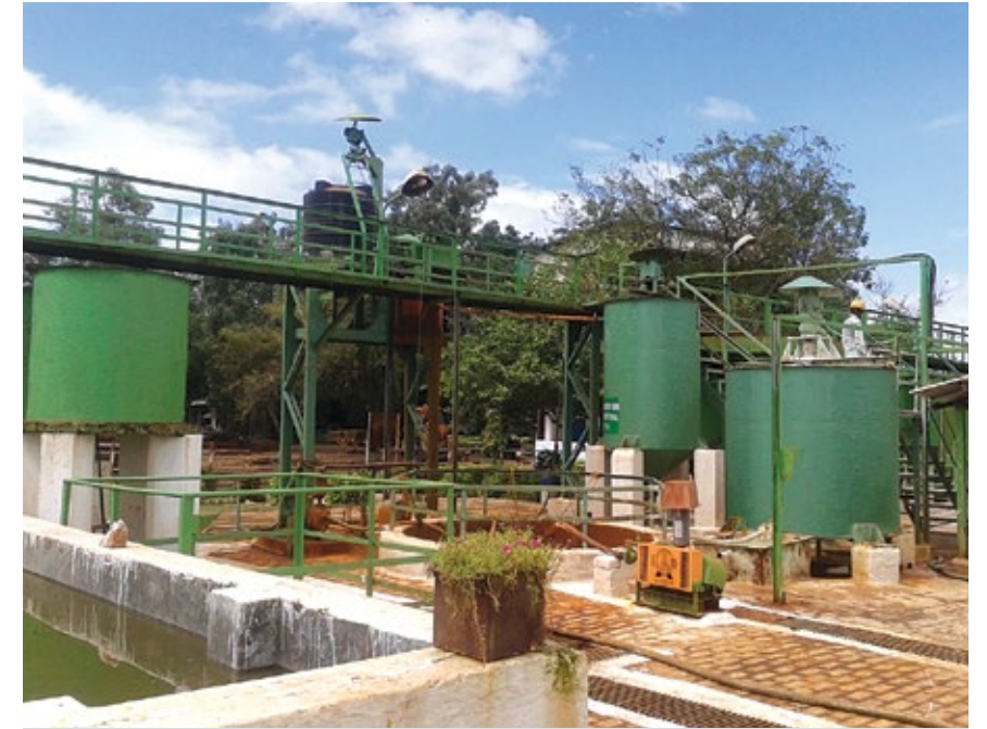
ETP Plant for spent acid neutralisation, Jabalpur
