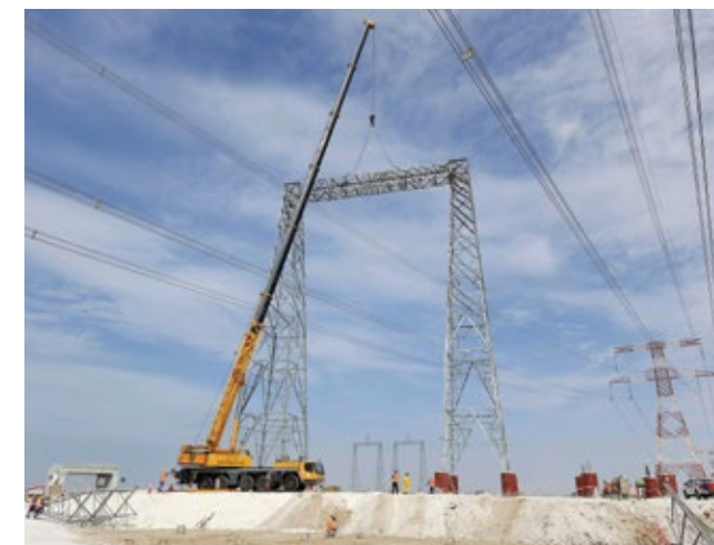
400 kV Transmission Line Project, Abu Dhabi, UAE
