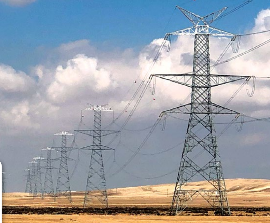
400 kV Atarat Oil Shale-Queen Alia Twin Conductor Transmission Line, Jordan
