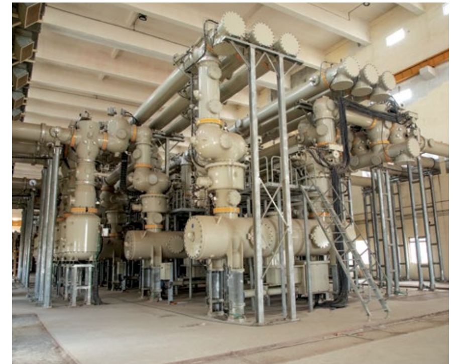
765/400 kV North Chennai Gas Insulated Substation, Tamil Nadu
