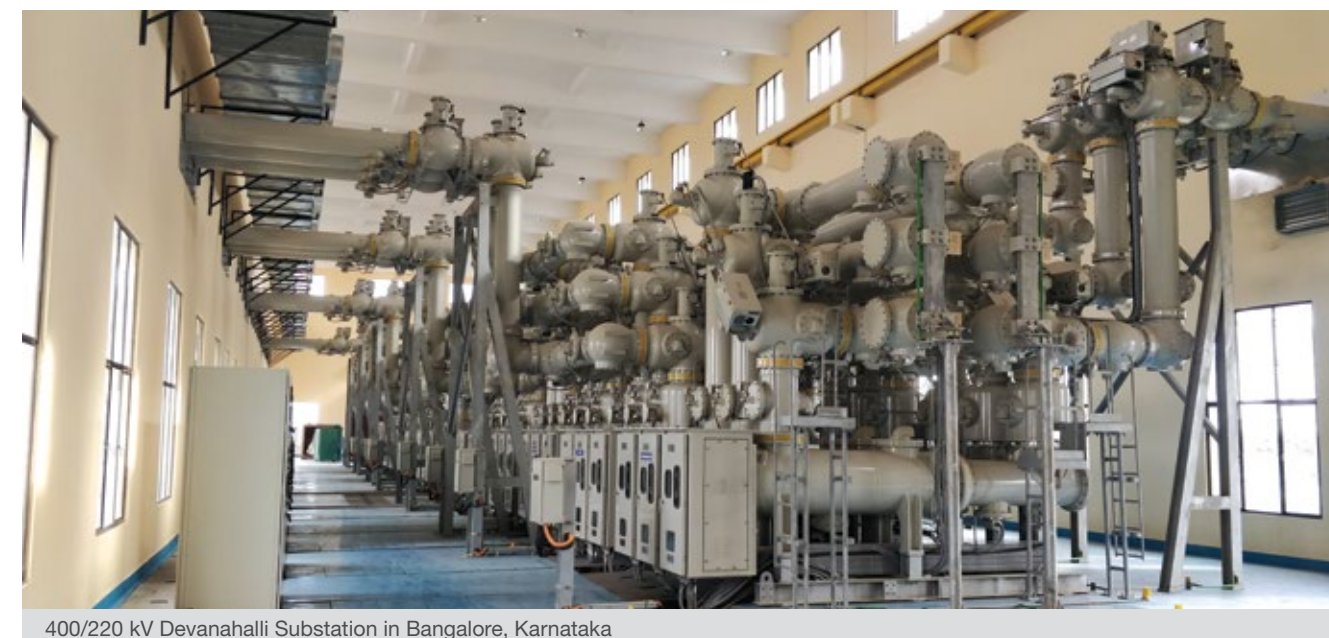
400/220 kV Devanahalli Substation in Bangalore, Karnataka
