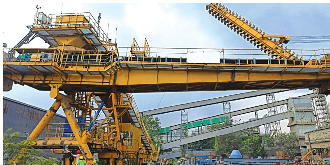
Erection & commissioning of Stacker and Reclaimer at a cement plant in Jamshedpur, Jharkhand
