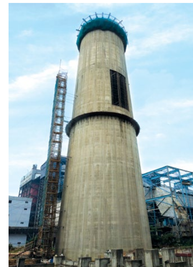
120-metre chimney at Flue-Gas Desulfurisation project, constructed through slipform technology, at Dhanbad, Jharkhand
