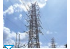
400 kV Pavagada - Devanhalli Transmission Line, Karnataka
