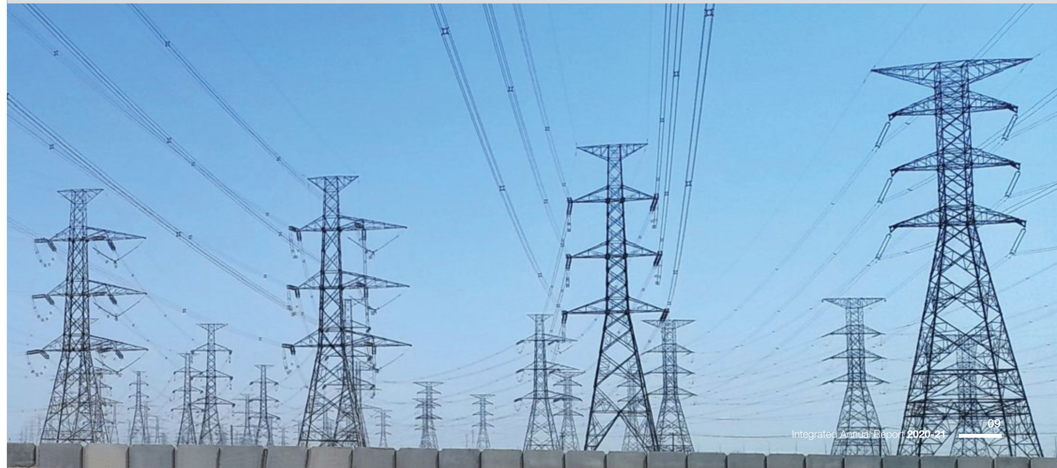
380 kV Transmission Line, Saudi Arabia
