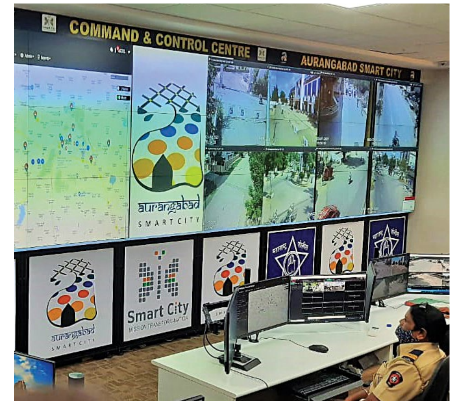
Command and Control Centre at Aurangabad Smart City, Maharashtra
