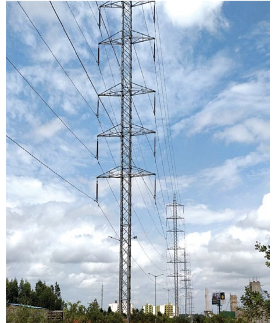
Narrow base towers
