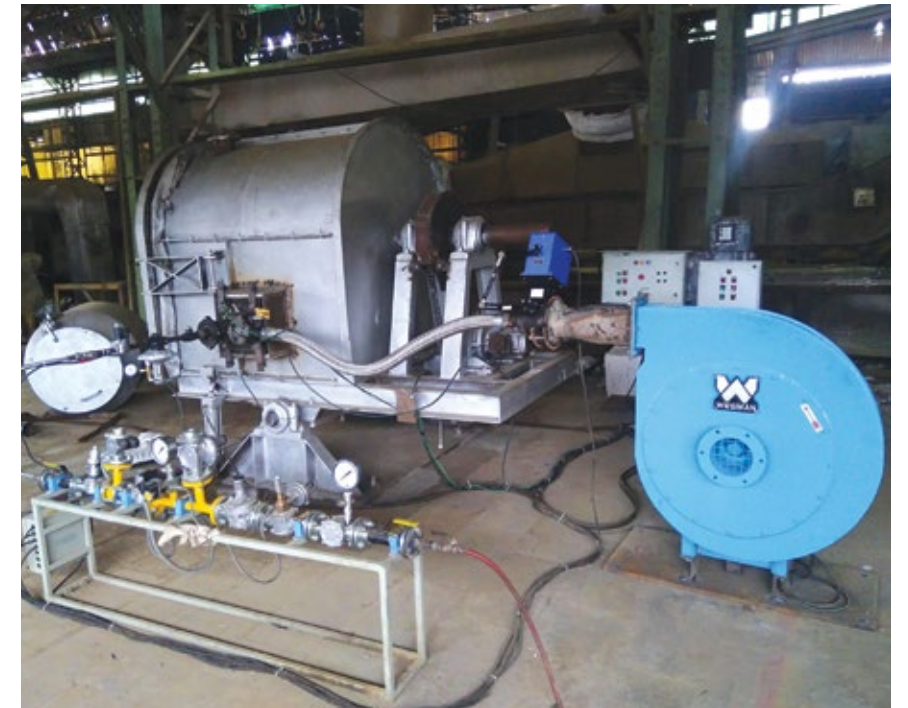
Zinc Recovery Furnace, Jabalpur
