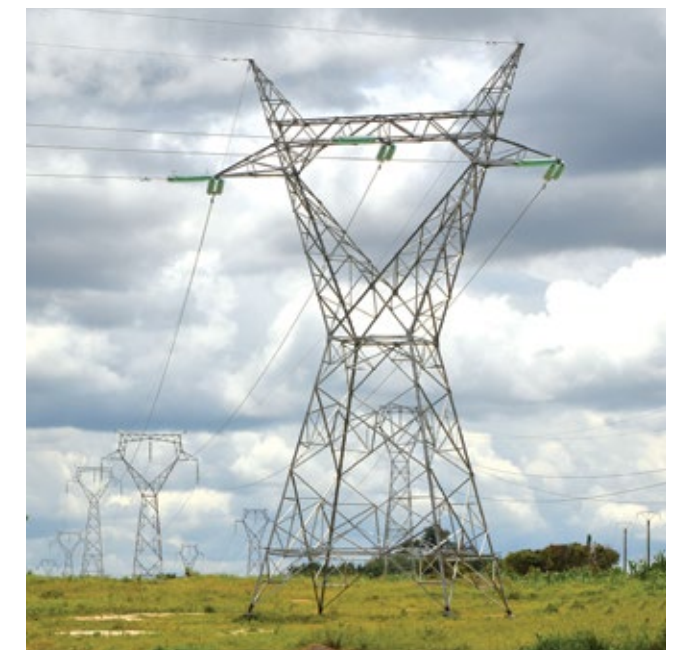
225 kV Transmission Line, Ivory Coast
