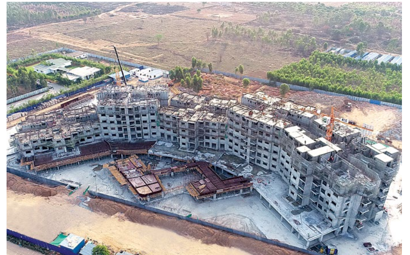
Construction of high-rise residential towers using aluminium formwork technology, at Bangalore, Karnataka
