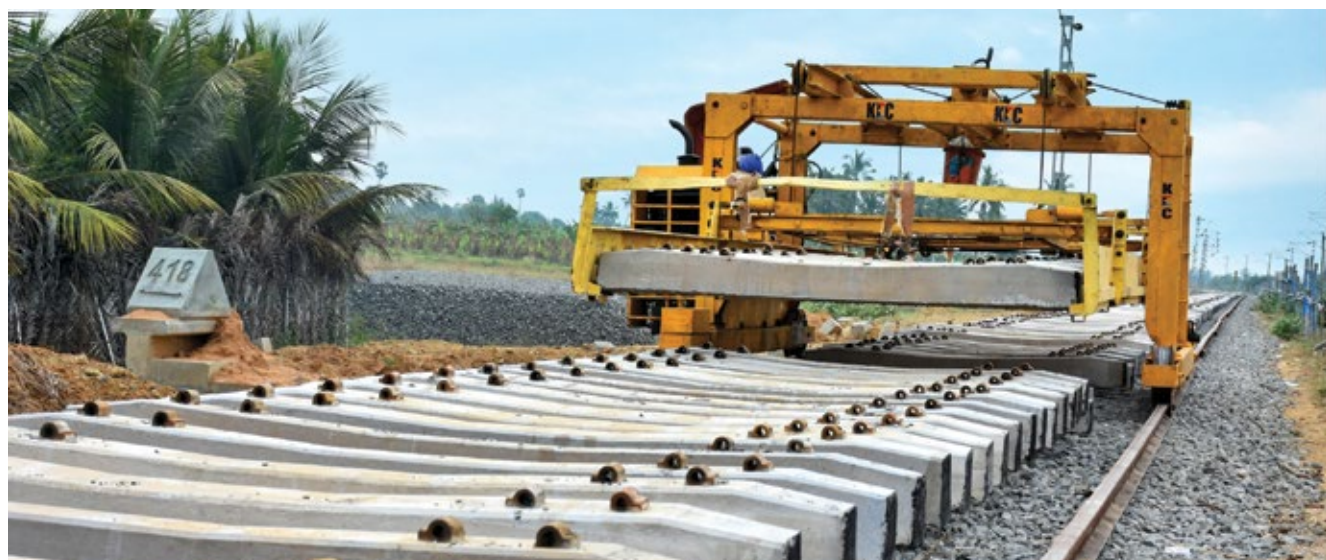
Sleeper Laying Machine at Vanchi-Maniyachchi (Nagercoil) doubling and overhead electrification project, Tamil Nadu
