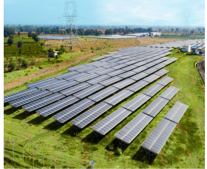
5.5 MW Solar Project
