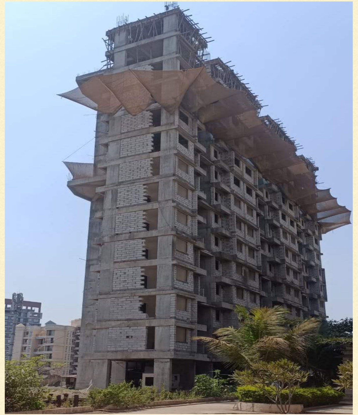
RCC work up to 14 th slab and finishing work till 10 th floor is in progress
