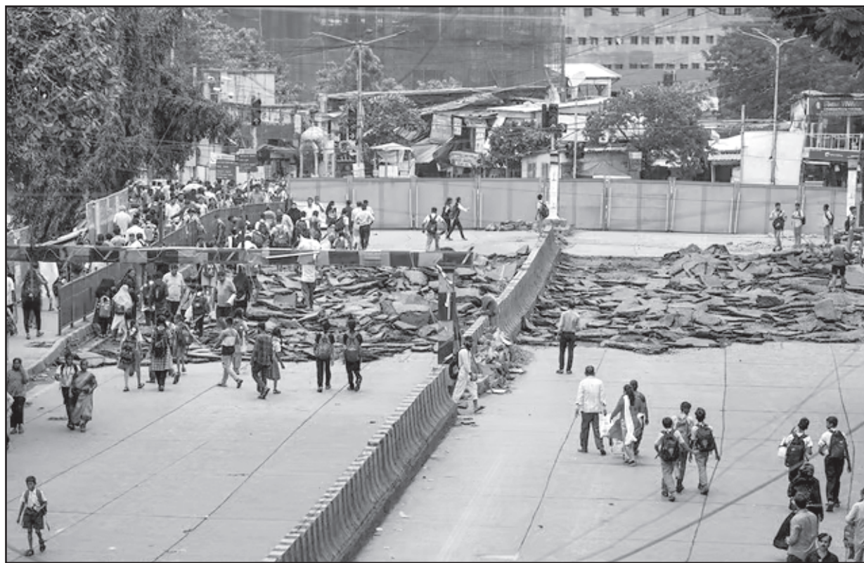
Old Sion bridge closed for demolition after the Indian Institute of Technology (IIT), Bombay, in its structural audit, had recommended the dismantling of the 112-year old British-era structure, in Mumbai on Thursday.
