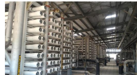
50 MLD BWRO (Desalination), for Reliance Industries, Dahej, India Turnkey project executed in record 8 months 24 days
