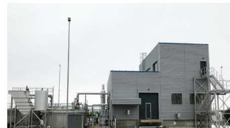
Industrial Effluent Treatment Plant for Phillip Morris, Otopeni, Bucharest, Romania Treatment of effluents from tobacco production
