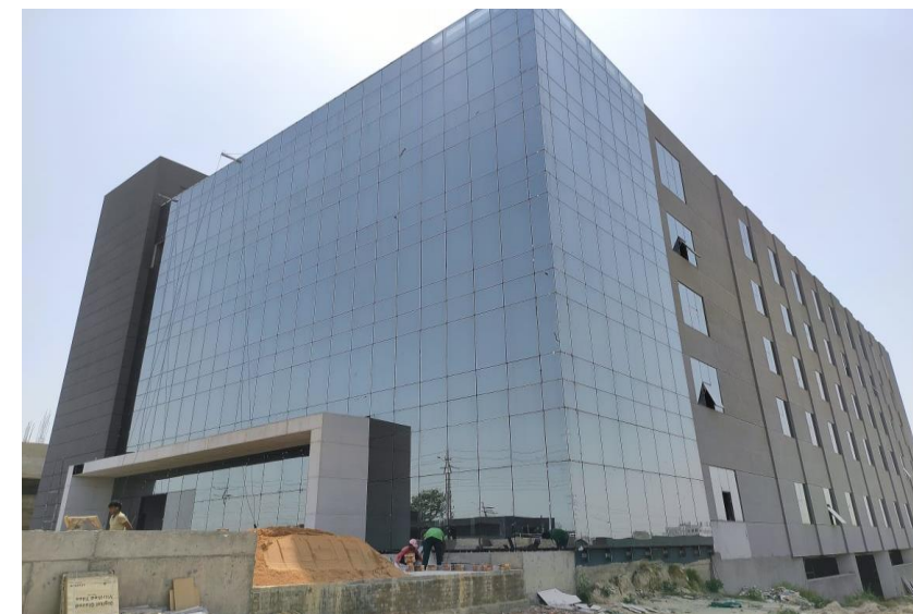
Site Pictures: Block I at Plot No 10, Sector 156, Noida, Gautam Budh Nagar, Uttar Pradesh
