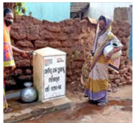
Su-Swasthya safe drinking water pipelaine, Sukinda
