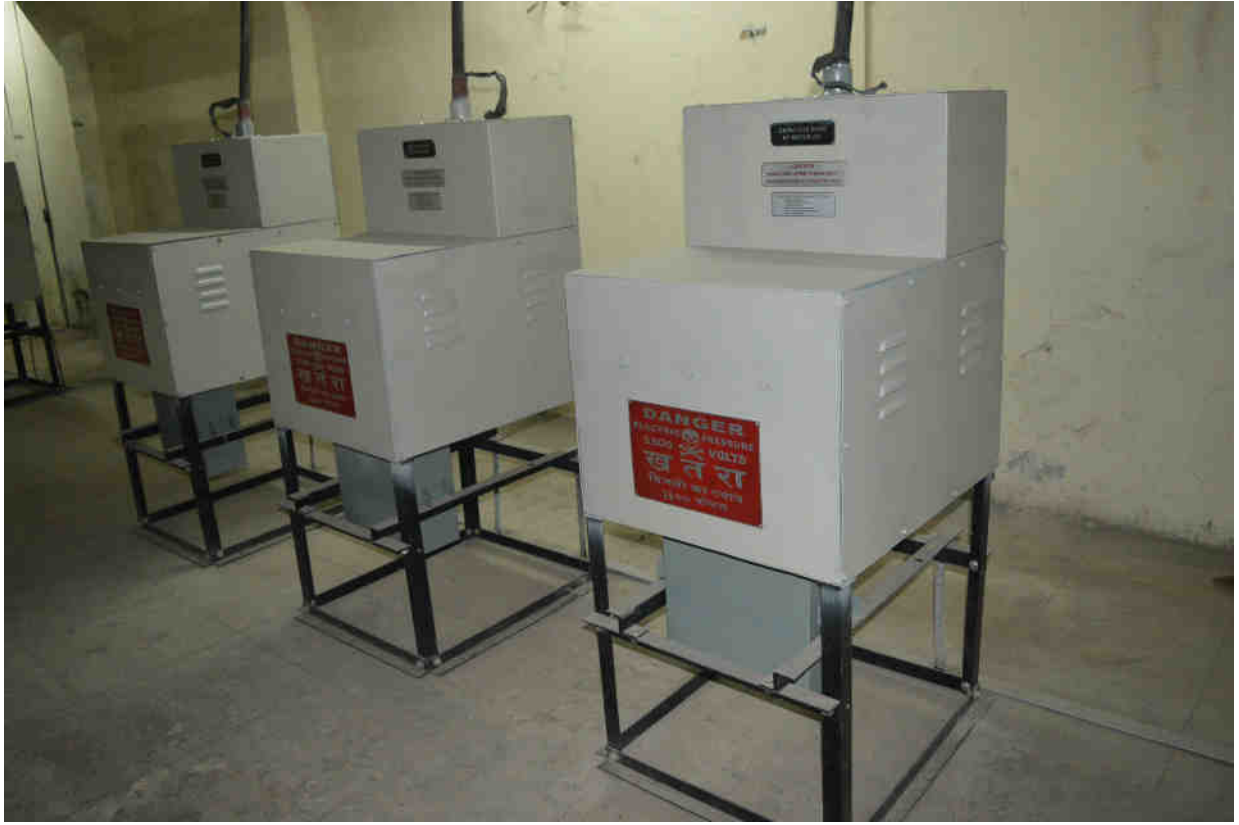
HT CAPACITORS CONNECTED ACROSS LARGE MOTORS
