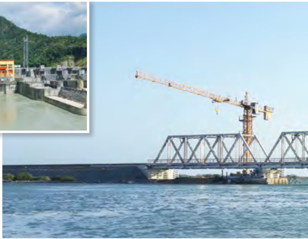
Railway Bridge in Jaffna, Srilanka (Total spans 3 x 37 meters) being manufactured & commissioned by Texmaco
