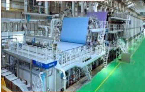
FINISHED PAPER – 1,82,400 TPA
