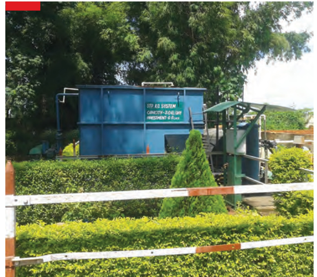
▲ STP plant for waste water treatment
