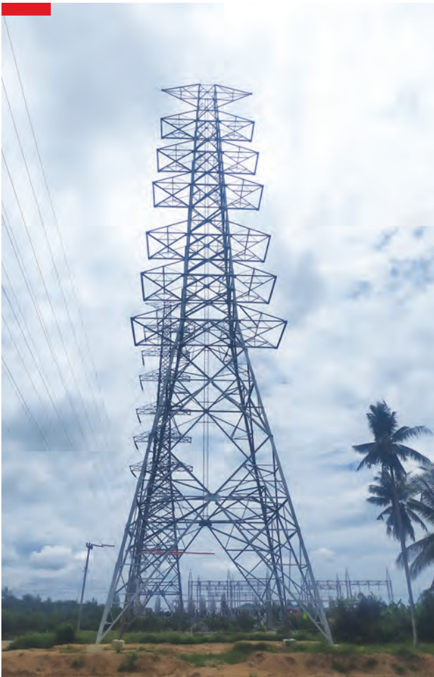
▲ 500 kV Transmission Line, Thailand
