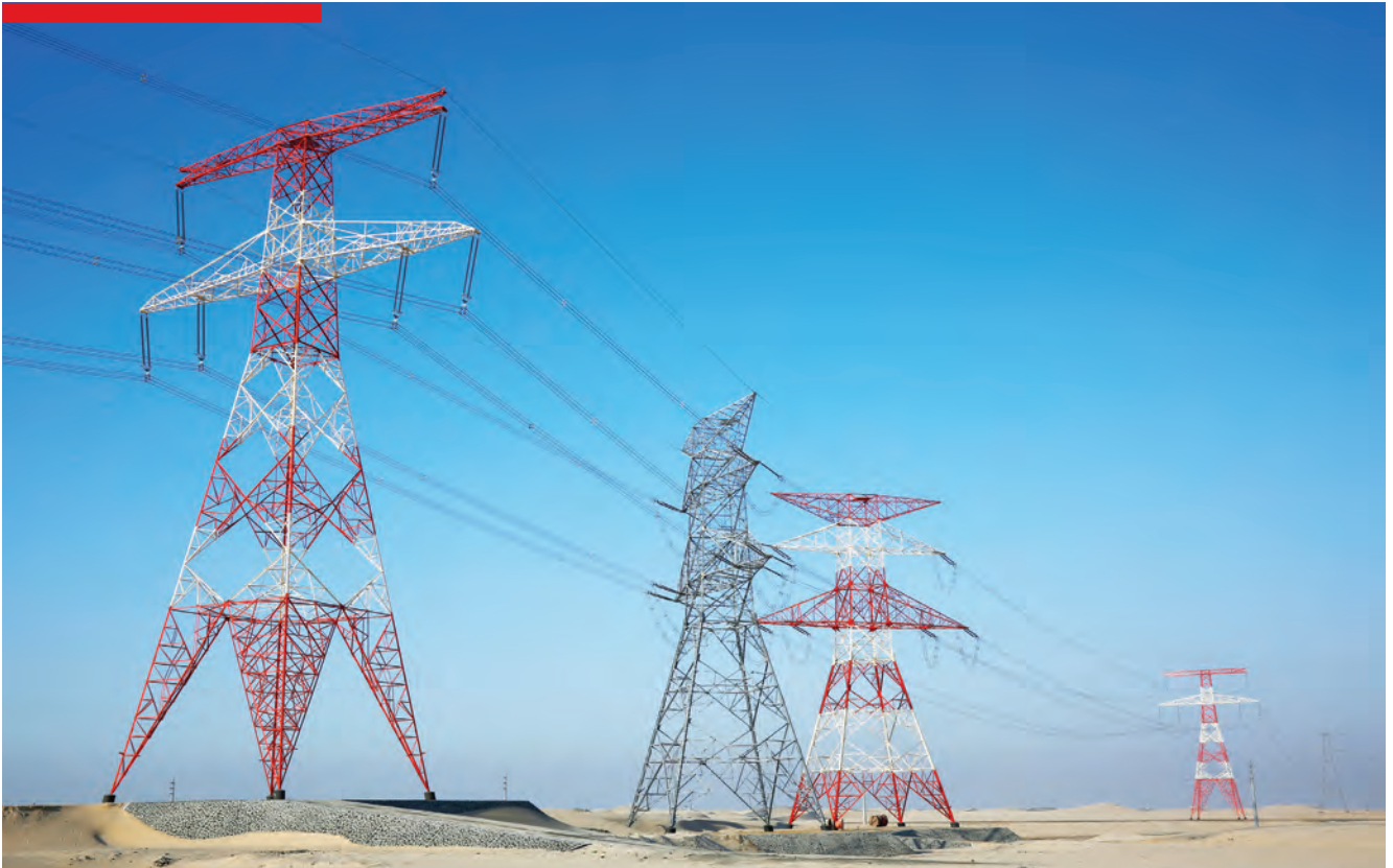
▲ 400 kV Overhead Transmission Line at Abu Dhabi, UAE
