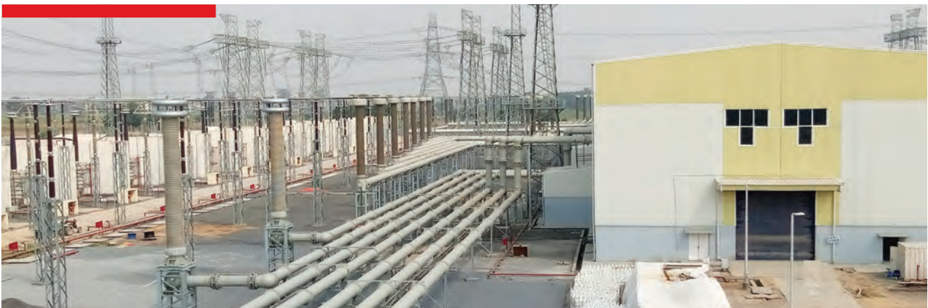
▲ 765 kV Gas Insulated Substation at Aligarh, Uttar Pradesh
