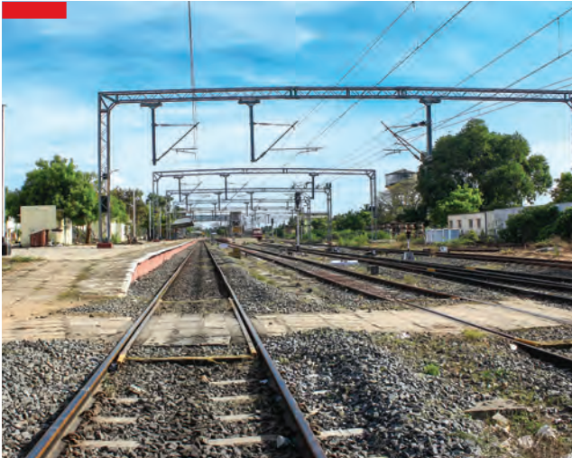
▲ Overhead Electrification at Villupuram, Tamil Nadu
