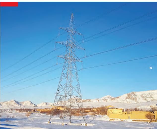
▲ 220 kV Ghazni-Kandahar Transmission Line, Afghanistan
