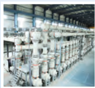
765/400 kV Gas Insulated Substation in Koteshwar, Uttarakhand
