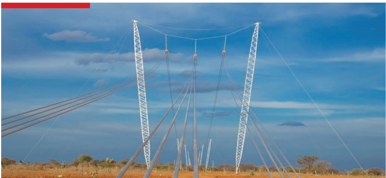
▲ 230 kV Rio Grande – Barreiras I – Barreiras II Transmission Line, Brazil
