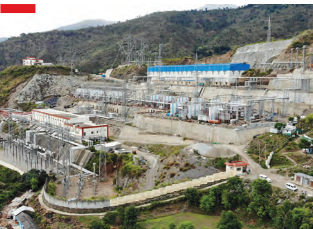
▲ 765/ 400 kV Gas Insulated Substation at Koteshwar, Uttarakhand
