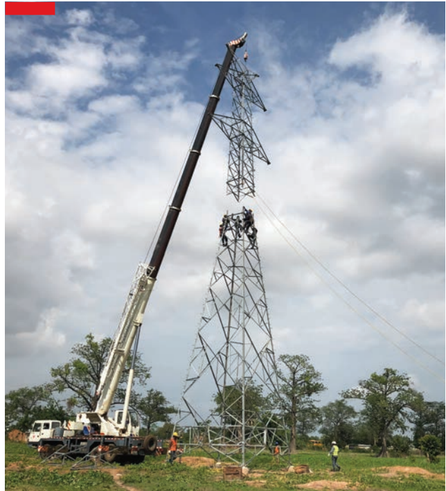
▲ 330 kV Kintampo-Tamale II Transmission Line, Ghana
