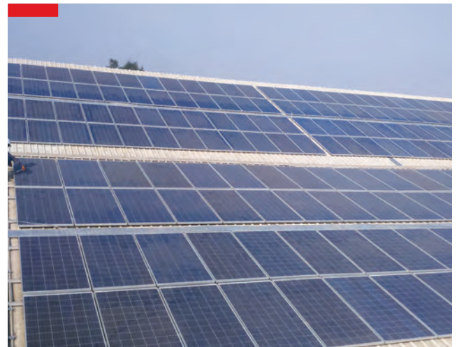
▲ 250 kW solar rooftop power plant, Butibori
