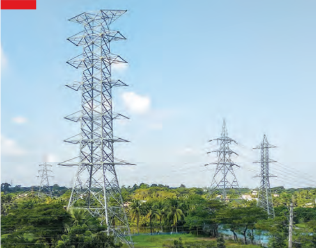
▲ 230/ 132 kV Transmission Line (Western Zone), Bangladesh
