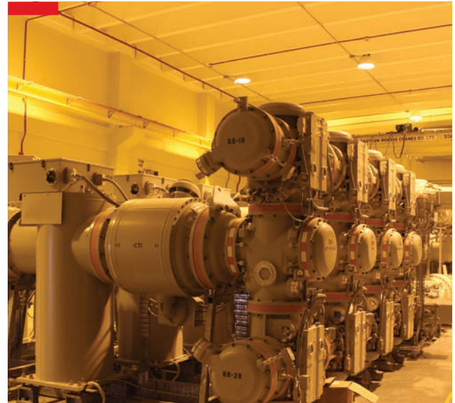
▲ 115/ 13.8 kV Gas Insulated Substation at Ain Murjan, Saudi Arabia
