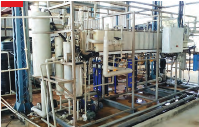
▲ Acid Recovery Plant, Butibori
