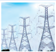
765 kV Fatehgarh-Bhadla Transmission Line, Rajasthan
