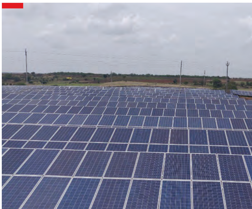
▲ 14 MW Ground Mount Solar project, Maharashtra
