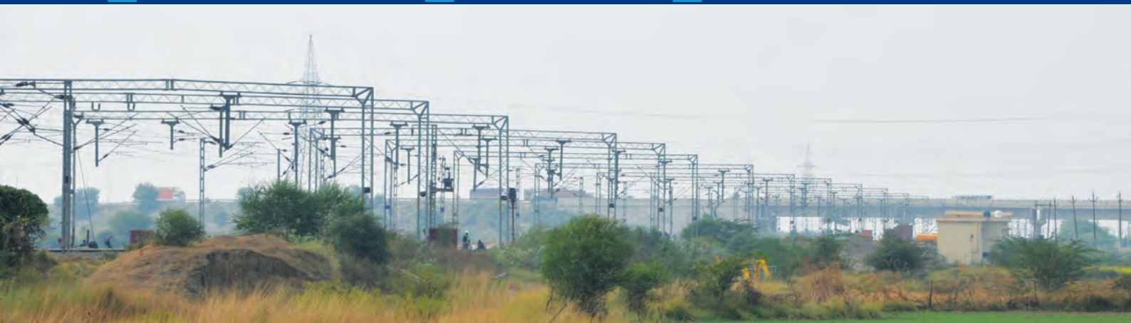
▲ Overhead Electrification between Jhansi-Bhimsen, Uttar Pradesh
