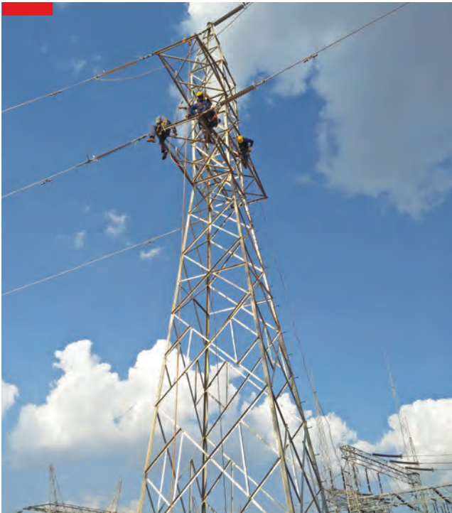
▲ 132 kV Mpanshya–Chitope Overhead Transmission Line, Zambia
