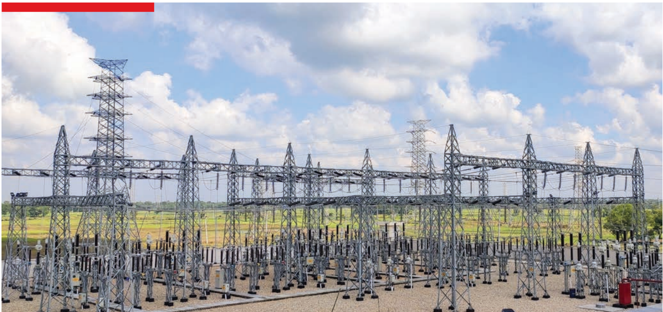
▲ 132 kV Air Insulated Substation at Chowddagram, Bangladesh; part of the six substation package for PGCB
