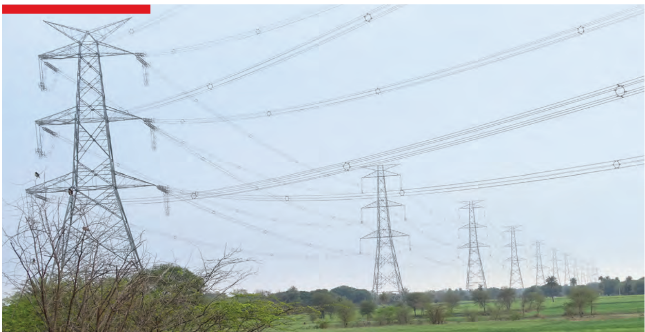
▲ 765 kV Banaskantha-Chittorgarh Transmission Line, Rajasthan; part of the Green Energy Corridor
