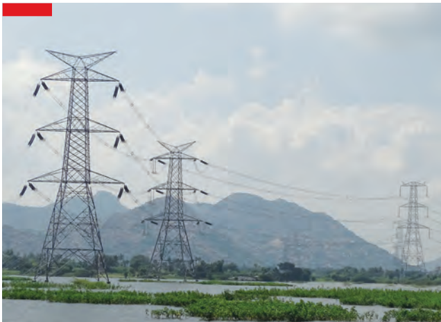
▲ 765 kV Ariyalur Transmission Line, Tamil Nadu
