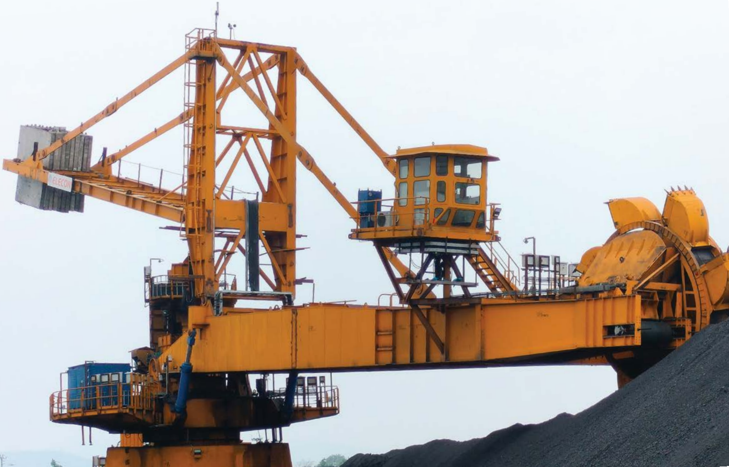
▲ Bucket Wheel type Stacker cum Reclaimer having capacity of 1200 TPH for CHP at MPPGCL, Birsinghpur, MP
