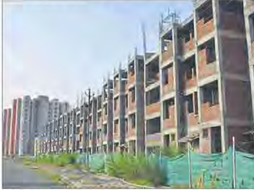
Builders seek the reiteration of a new scheme for the urban middle-class population would boost the confidence of both the common man and the real estate sector.
