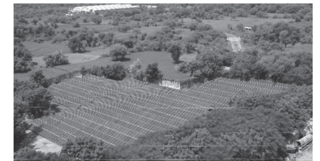
500 KW Solar Power Plant at Kalol, Gujarat
