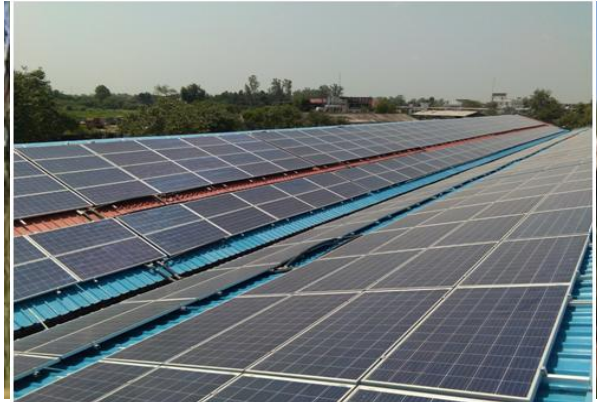
UPA Ltd – Solar installation, UP.
