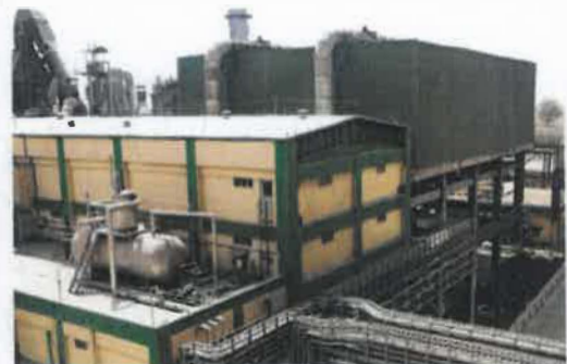
Waste Heat Recovery System
