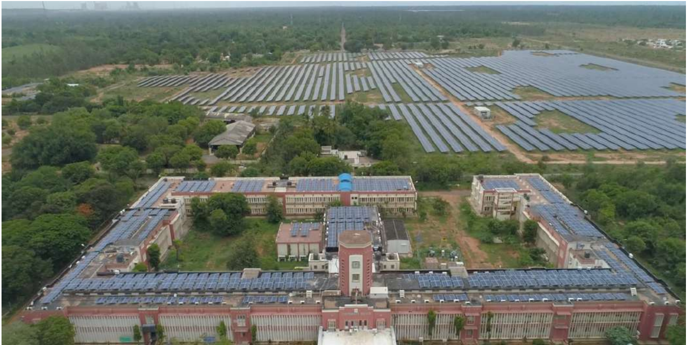
Rooftop Solar Plant at Corporate Office, Neyveli
