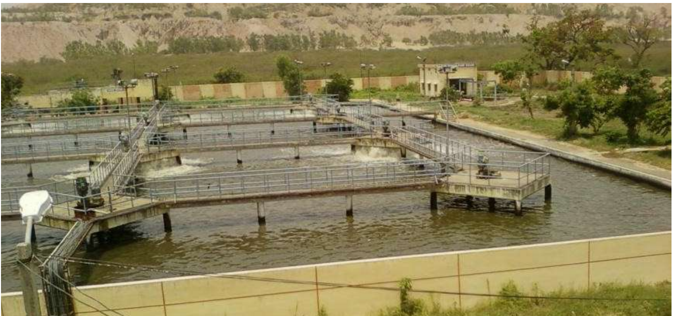
Municipal Sewage Treatment Plant – Neyveli Township
