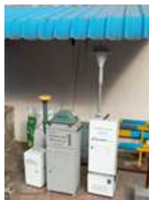
AAQ Station installed in Vadakuvellore, Neyveli
