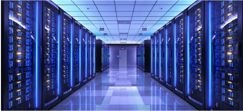
Compact substations, smart power products, MV switchgear for a large data center project
