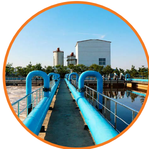
Miner & Irigation Department UP Project-Water distribution Products Used-MS Pipes
