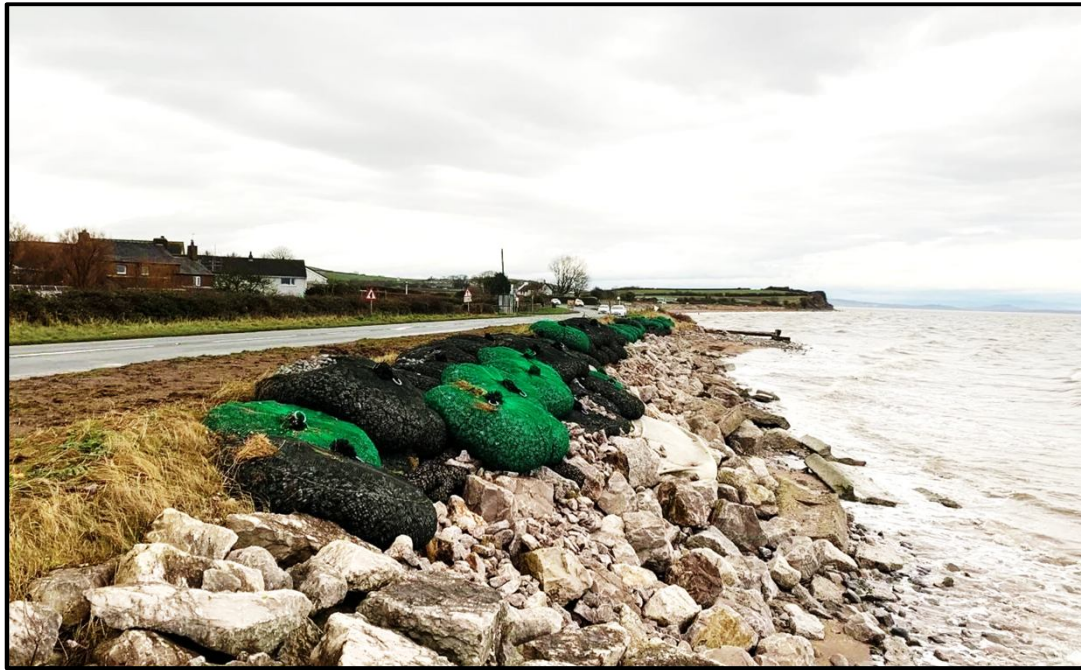
Erosion Control and Scour Protection along a coastal road in Cumbria, North England
