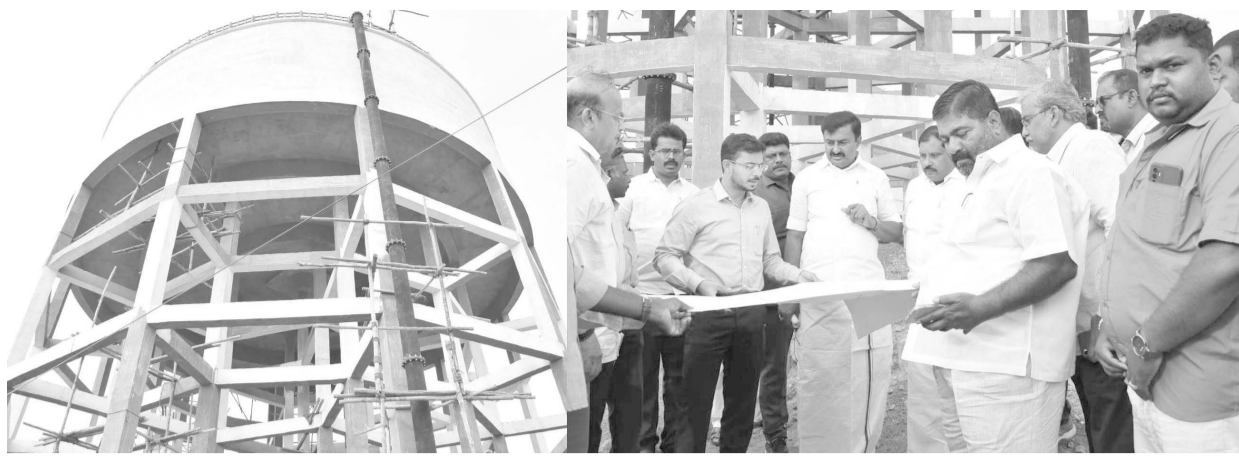
Tamil development and publicity minister MP Saminathan inspected the construction works of an overhead tank with a capacity of 10 lakh litre under water augmentation scheme at Sneh Nagar in Tirupur district. Collector Christu Raj, city mayor Dinesh Kumar, corporation commissioner Pavankumar G Giriyanavar, deputy commissioner Balakrishnan, corporation zonal chairpersons Padmanaban and Govindarajan, and others were present at the venue.
