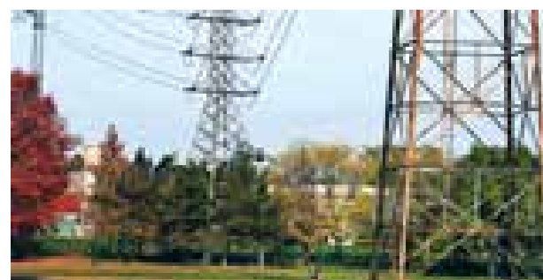
Uttarakhand Power Corporation Limited (UPCL) Project: Rural Electrification Products Used: Steel Pipes & Steel Poles
