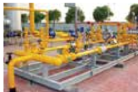
Gujarat Gas Limited Project: Gas distribution Products Used: Pipes
