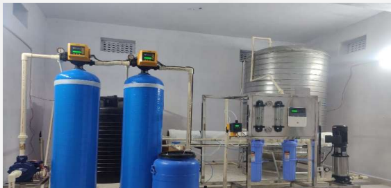
Setting up of R O Water Plant at Kakinada District of Andhra Pradesh.
