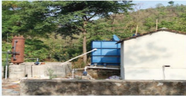
Setting up of Water Treatment Plant(WTP) & Sewage Treatment Plant (STP), Om Creations Trust, Maharashtra
