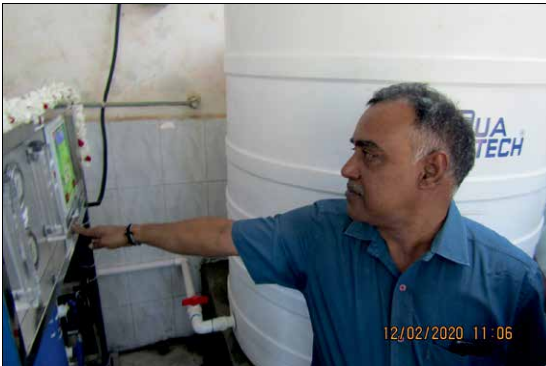
RO plant at Kalapet girls school
