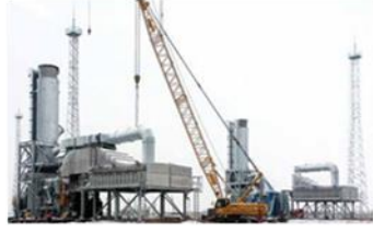
35 MW GT POWER PLANT, KAZAKSTHAN
