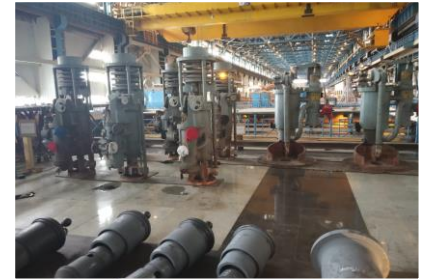
CONTROL & STOP VALVES OVERHAULING SIPAT 660MW
